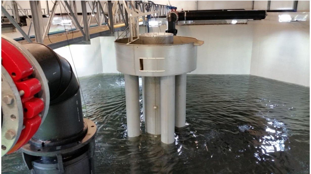
Figure 5. A center drain and mortality collection apparatus is exposed as water and fish are pumped from a smolt tank to a central vaccination station at the Marine Harvest Steinsvik hatchery. The vertical pipes impact water rotation and mixing about the center of the tank.
